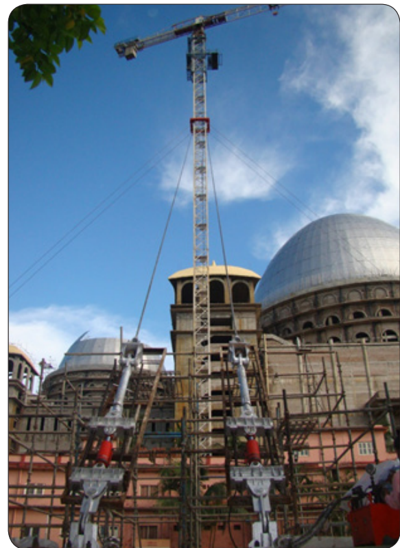
Tower Crane Anchoring System
