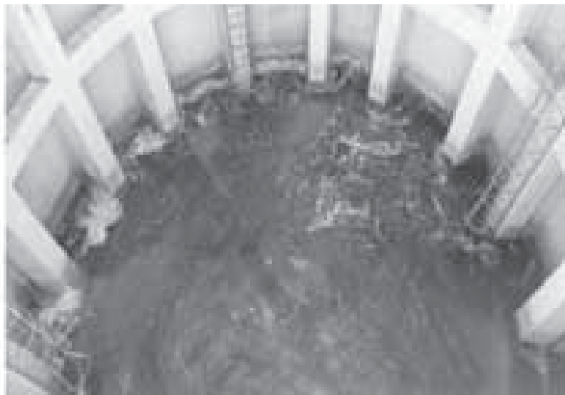
Intake Well, Kalpakkam, Tamil Nadu
