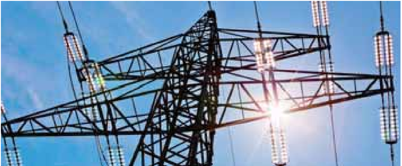
400 Kv Transmission Towers
