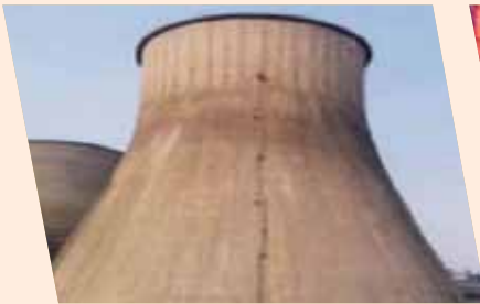
Tallest cooling tower of 141 metres at Panipat, Haryana, in 2000, the tallest in India at that time
