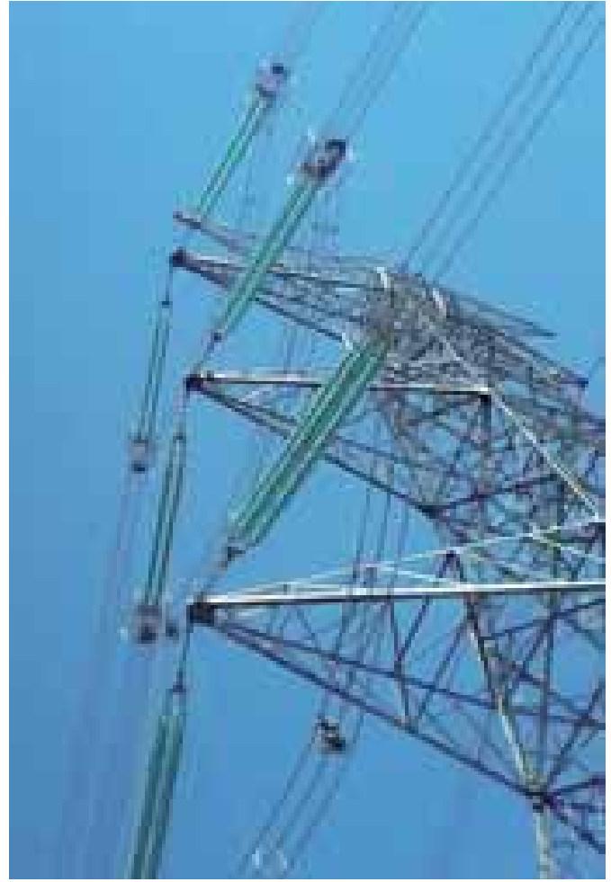
765 KV DC Wardha-Raipur Transmission Line
