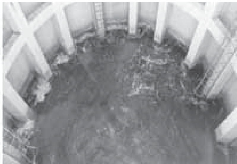
Intake Well, Kalpakkam, Tamil Nadu
