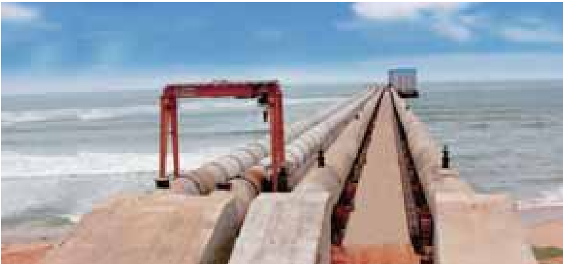
Hinduja Power Project, Vizag
