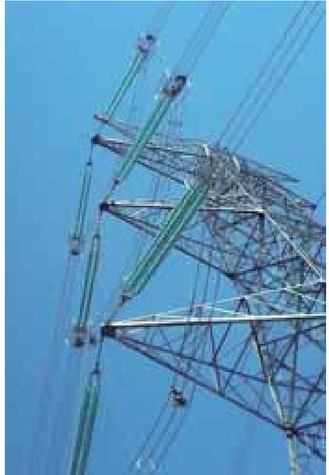
765 KV DC Wardha-Raipur Transmission Line
