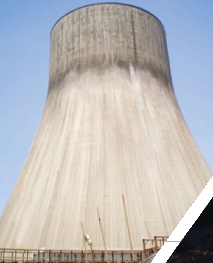
Cooling Tower, Bhusawal, Maharashtra
