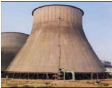
Tallest cooling tower of 141 metres at Panipat, Haryana, in 2000, the tallest in India at that time
