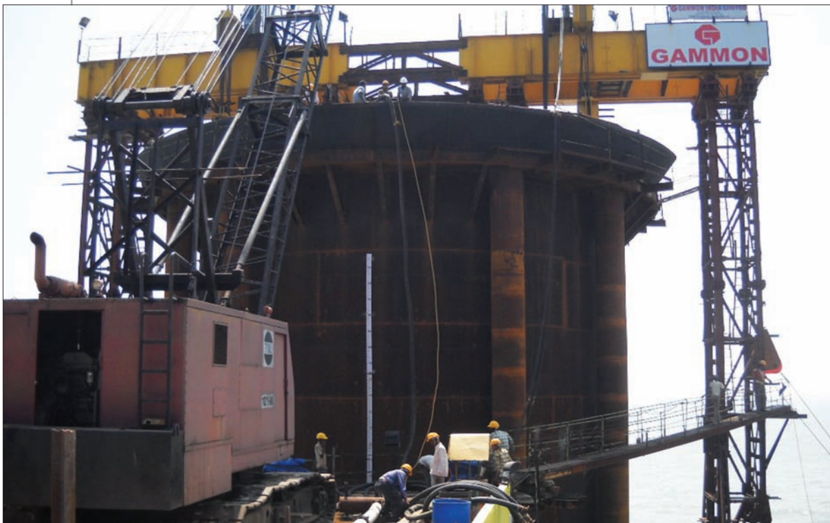
Kalpakkam site has completed the critical activity of caisson lowering and grounding for Sea Water Intake project. This is the first time Gammon has launched such a large caisson of 21 metres over cofferdam using latest technologies and a totally different technique that too in rough sea.
